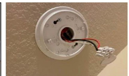
Baseplate only with missing detector unit
